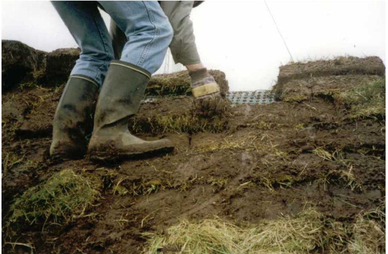
Fig. 15. The sods are laid bonded from the eaves upwards to the ridge. As the rows are completed, they are trampled firmly together.
