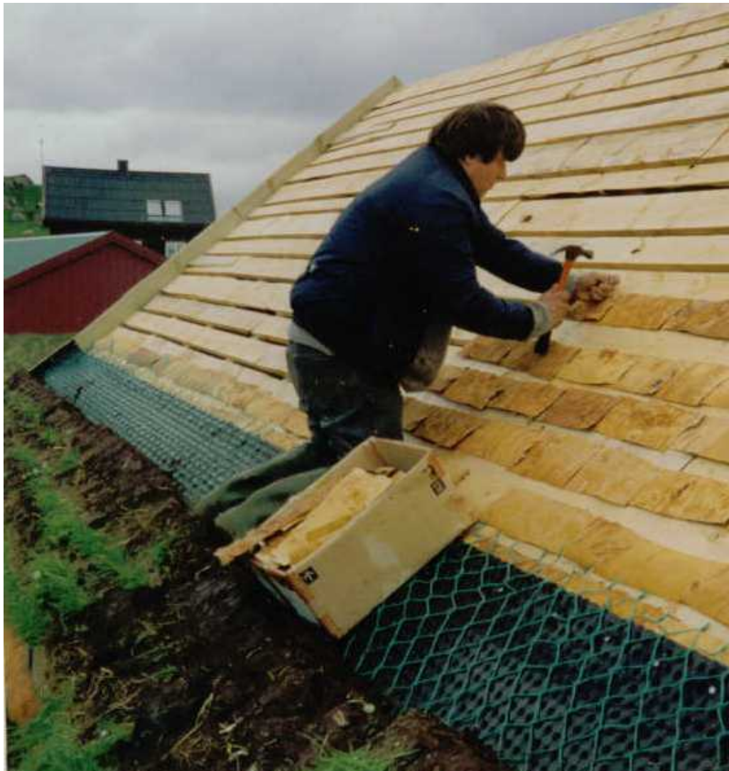
Fig. 20. Bark is only used where the base becomes visible, e.g. where the rafters or laths are spaced. The bark is laid on top of the laths in strips lengthwise along the eaves and protruding towards the drainpipe.
